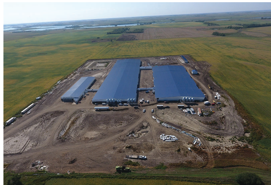
Above left, showcases an aerial view of the general layout of the farm along with the ongoing construction to finish up some other projects. On the right, the open pen gestation area is shown. There is a 16 square foot space for each sow. The sows have their own private space for the
