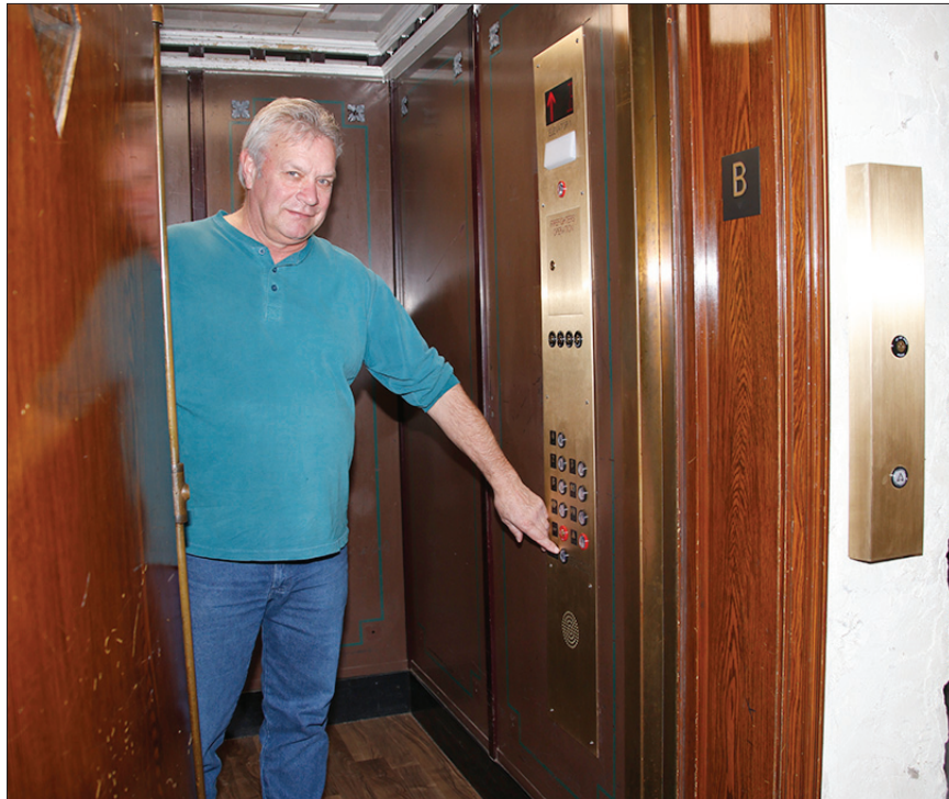
The elevator at the Clark County Courthouse may still look vintage, but its mechanics are new and state of the art with work being done recently to upgrade the elevator. Custodian Dustin Elsen points to the new phone system alarm button on the panel labeled 'help'.
