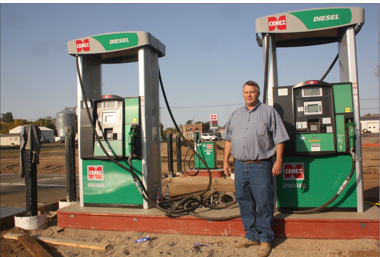
Clark Community Oil Company general manager Troy Grensberg is shown by the new diesel pumps on US Highway 212, in Clark. This renovation should be completed in the near future, allowing semi-trucks the
