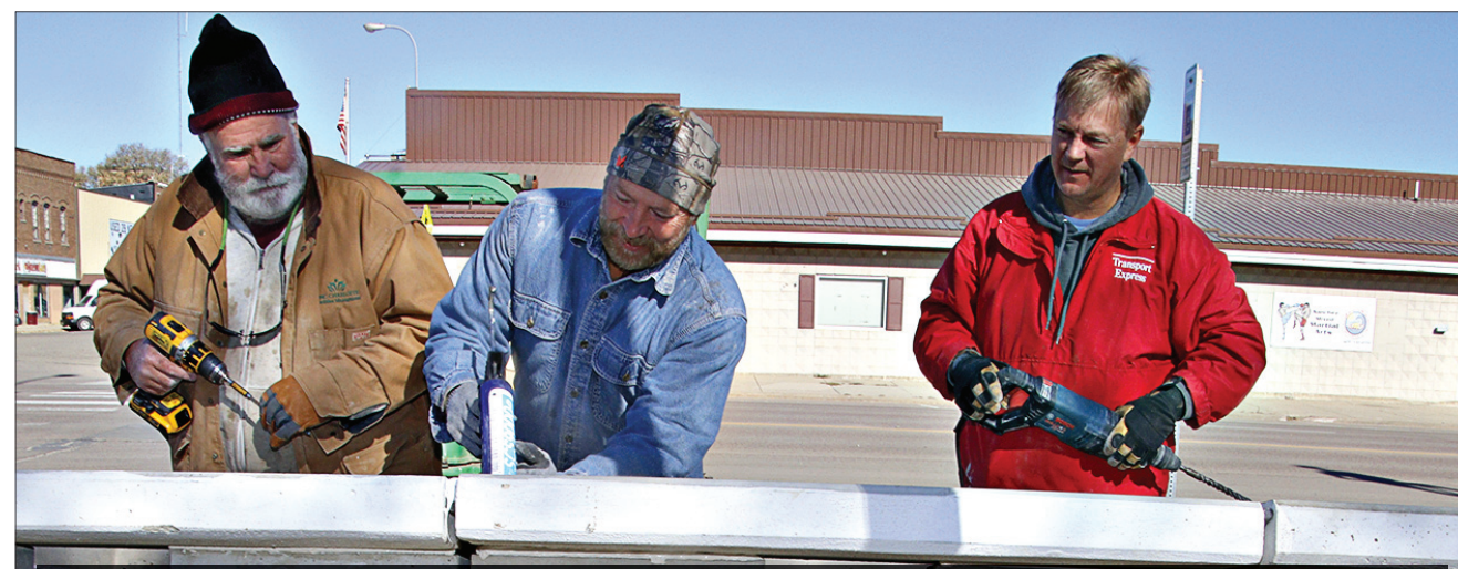
Don Ramsey, Darin Lewis and Dave Adam were working steady last Tuesday on the Charters of Freedom document chambers at Flat Iron Park in Clark. Each chamber will hold a 60 lb. bronze plate onto which the Declaration of Independence, the U.S. Constitution - in four sections and the Bill of Rights will be placed.
