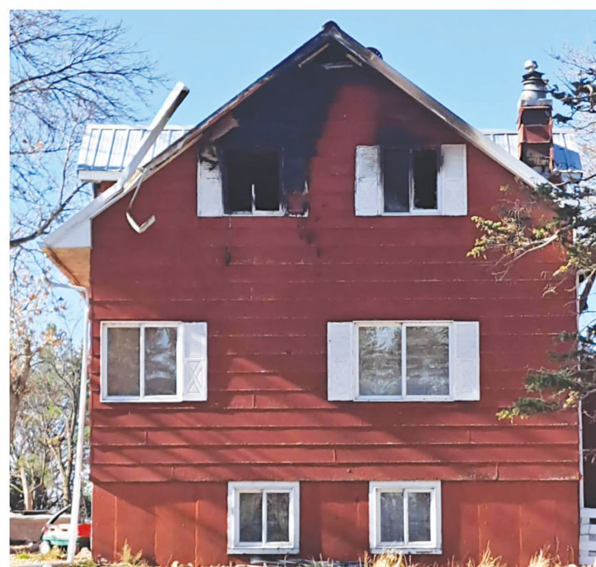
Pictured above is Bill and Jody Fuller's home southeast of Clark showing fire damage in the upper level. The blaze occurred Tuesday, November 5.
