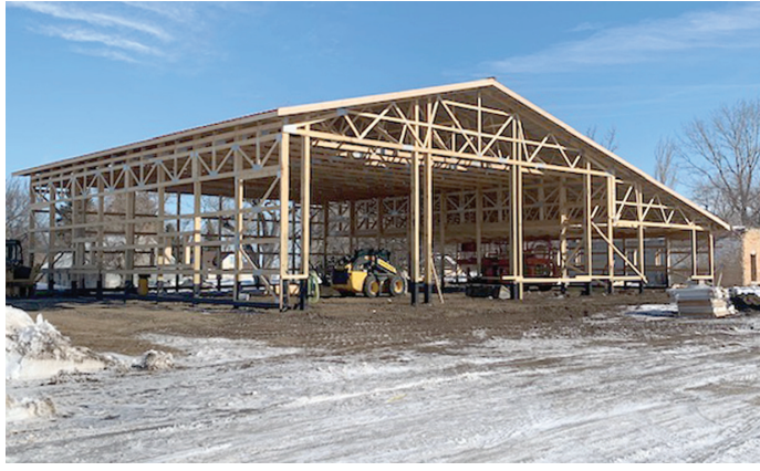
Pictured above is the outer shell of the new Garden City Fire Department that has recently been constructed. The building will also have a community room for local meetings and department trainings.
