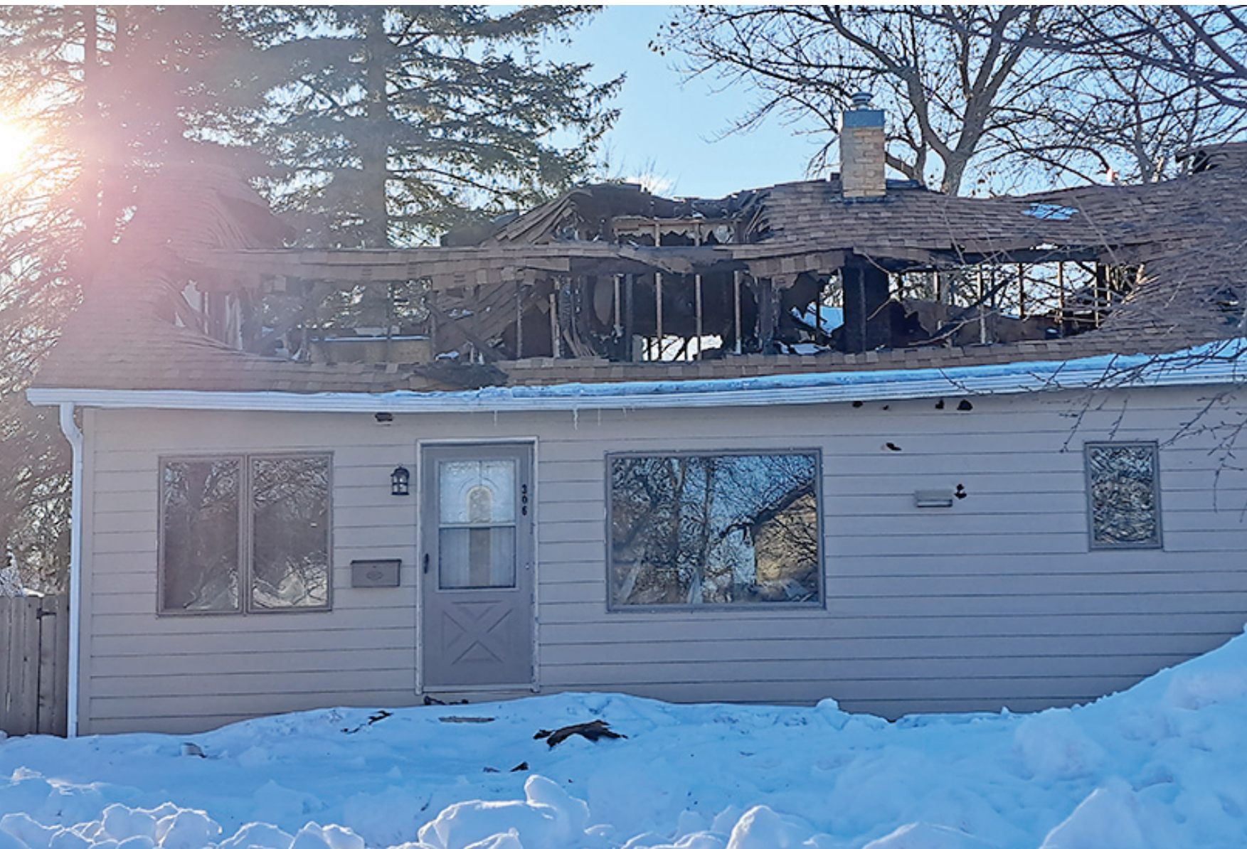
The picture above, taken Monday evening, shows the damage done to the house by the fire on Friday morning.
