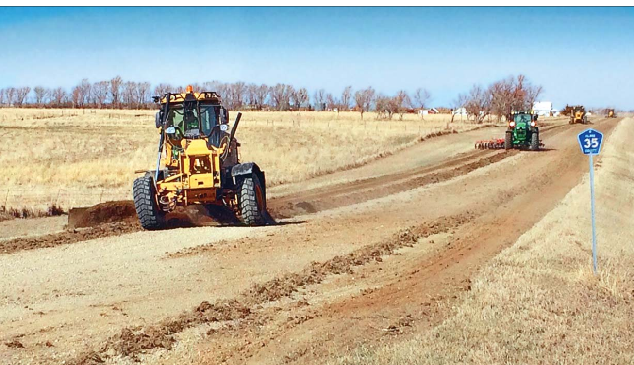
With less mud to deal with this spring, the Clark County crews have been busy 'pulling up the shoulders' on 70 miles of road. Shown above, three road graders with the help of a tractor and 12 foot offset disc, go along and pull over the gravel that has
