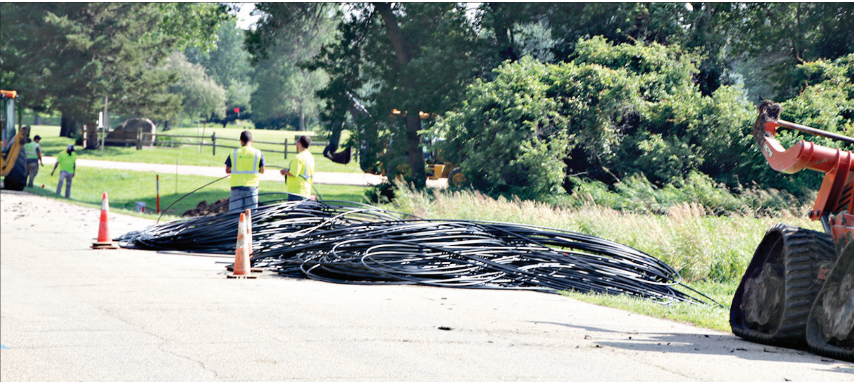
A huge amount of fiber optic cable was placed along Idaho Street in Clark this week as the project continues of burying the cable for Interstate Telecommunications Cooperative - or ITC.
