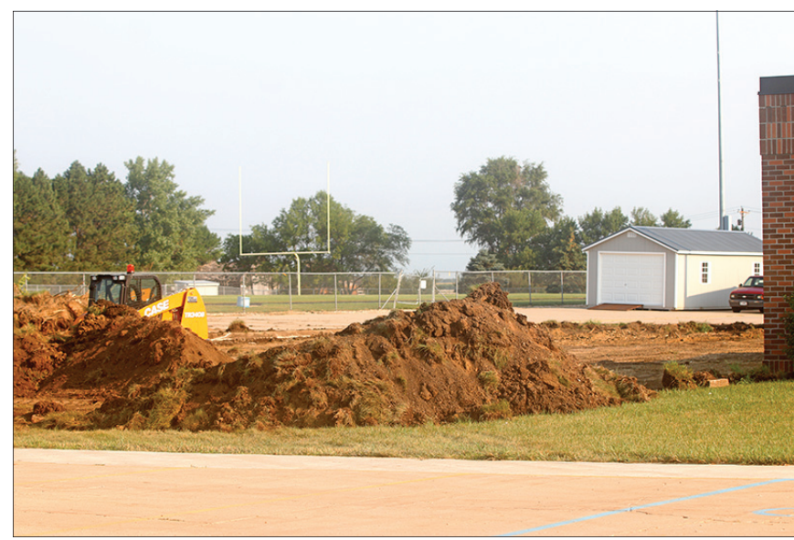
The concrete project on the west and south sides of Clark High School has begun.
